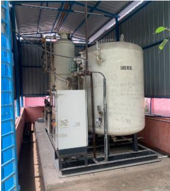
Image 2: Oxygen Plant in CHC Lalitpur
