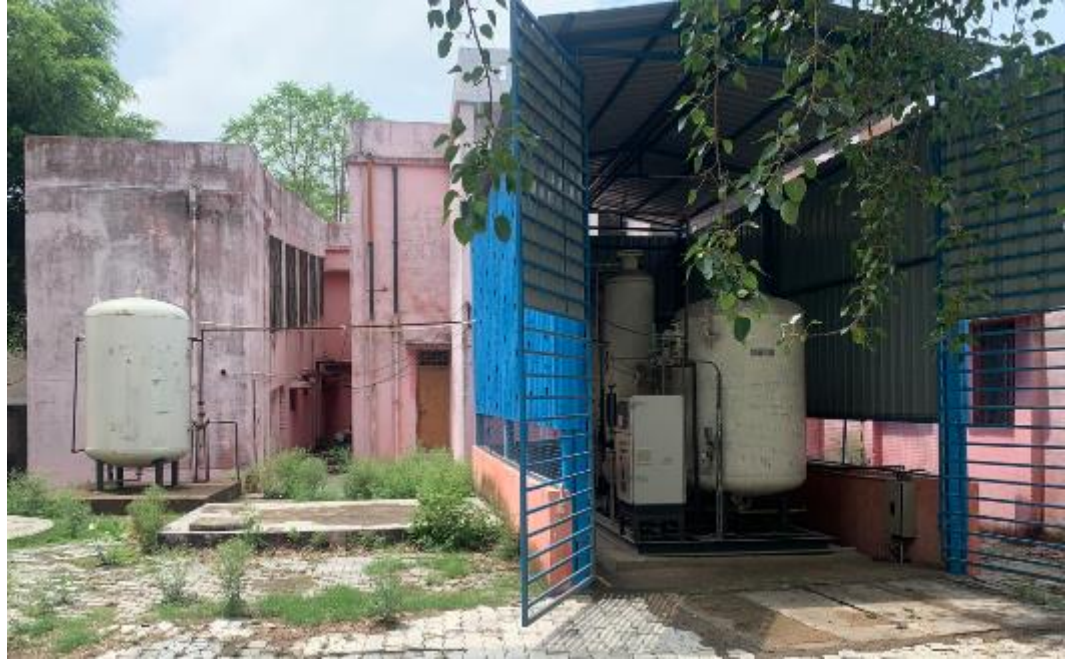
Image 3: Oxygen Plant installed in CHC Badagaon Jhansi
